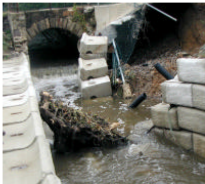
Creek Damage at Ridge Avenue
